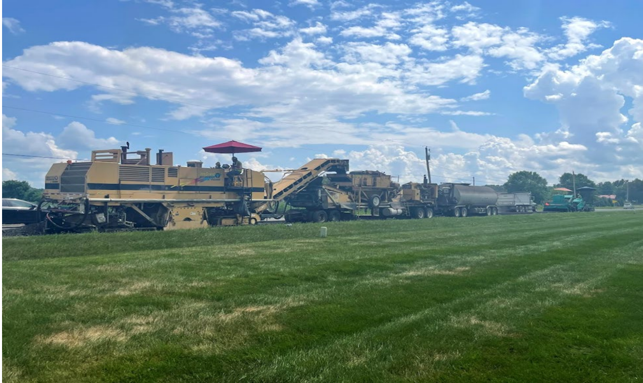
Figure 15 Multi-unit CIR Train (Courtesy HRG)
