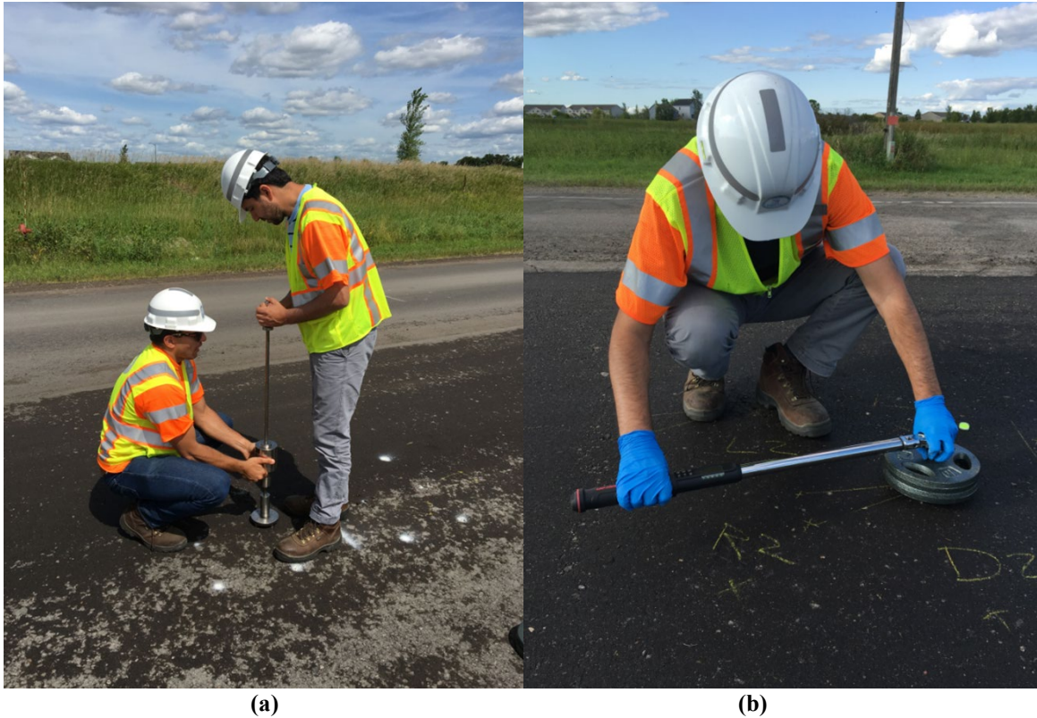
Figure 25. (a) Dynamic Cone Penetrometer weight being used to drive the long-pin shear device into the cold recycled mat while counting the number of blows and (b) torque being applied to the long-pin shear device and recorded.
