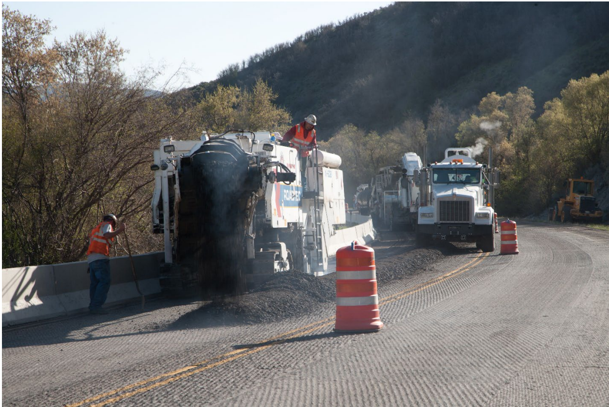
Figure 9 Recycling the shoulder plus full lane width by using a second milling machine. (courtesy ARRA)
